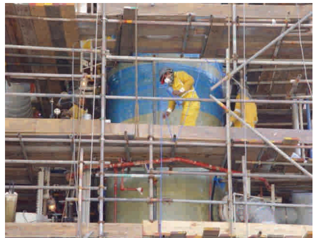
A repair applied to 2-meter diameter scrubber operating at 60 bar and 80°C
