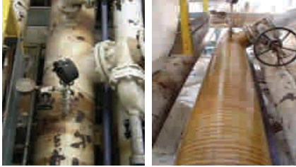
Before and after pictures of a 16-inch flare line operating at 7 bar and 2000C which had suffered internal erosion
